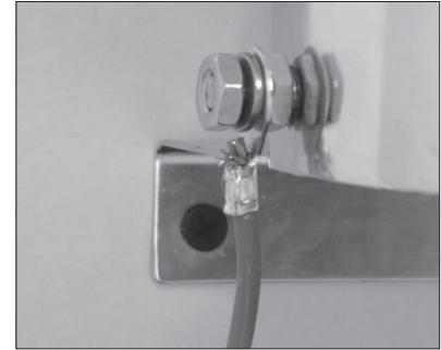
Photo 3 - Copper wire in contact with the screw and bolt on unit
